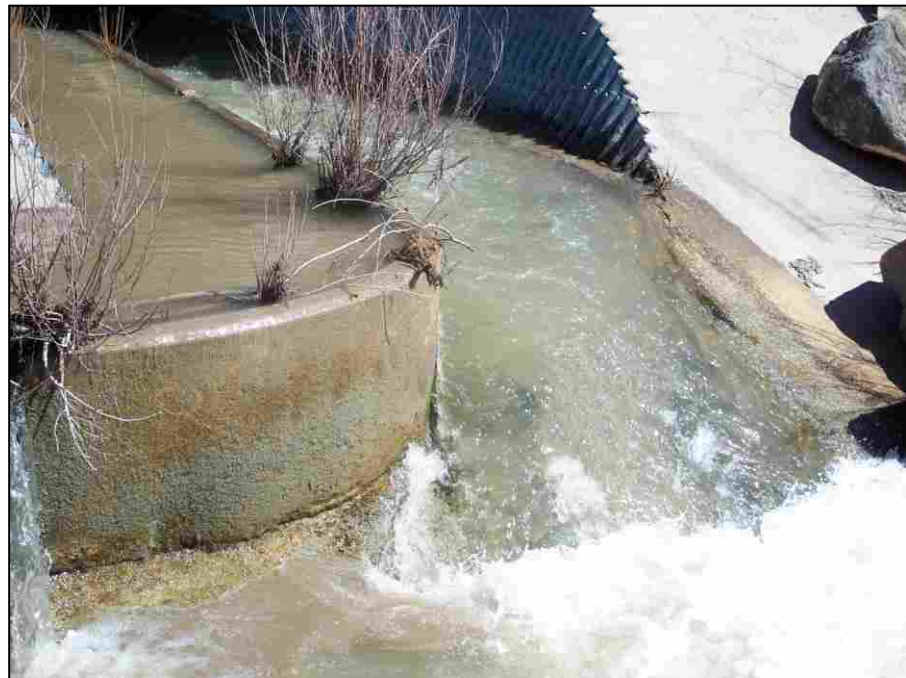
Figure 5-6: Photo of Discharge at Outlet Invert
