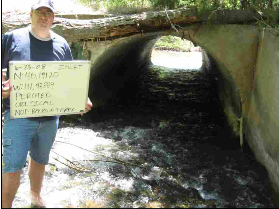
Figure 4-3: Hydraulic Evaluation Photo Taken at the Inlet
