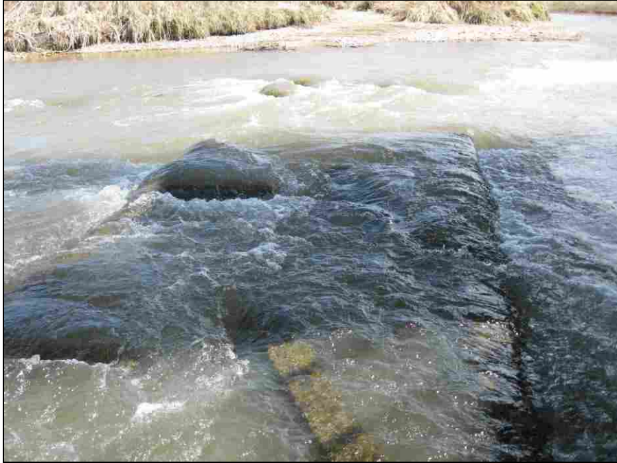
Figure 5-13: Photo of Fish Baffles at Inlet (Looking Upstream)
