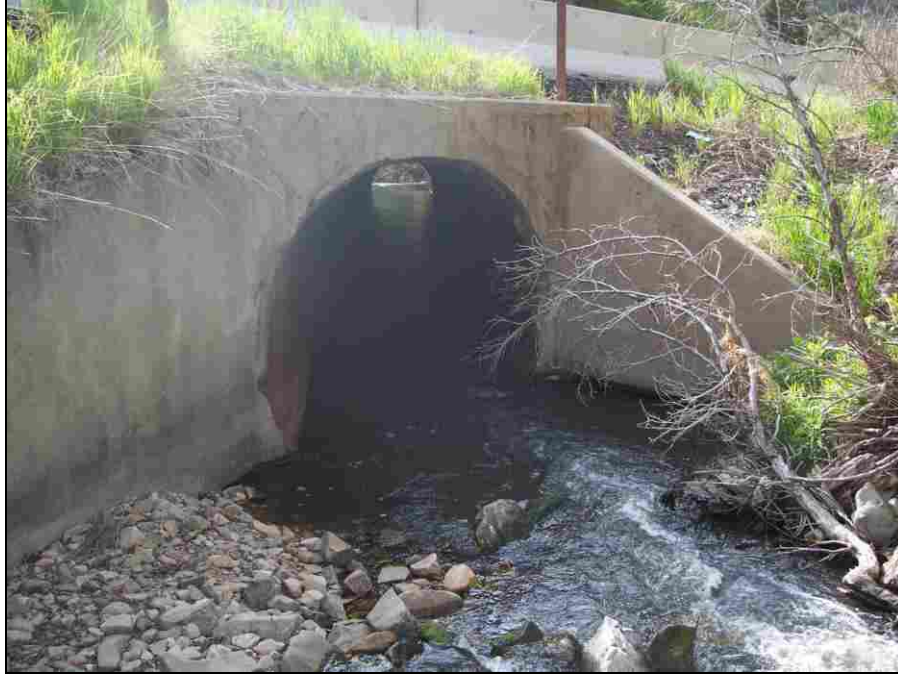
Figure 4-12: Inlet of Backwatered Culvert #3
