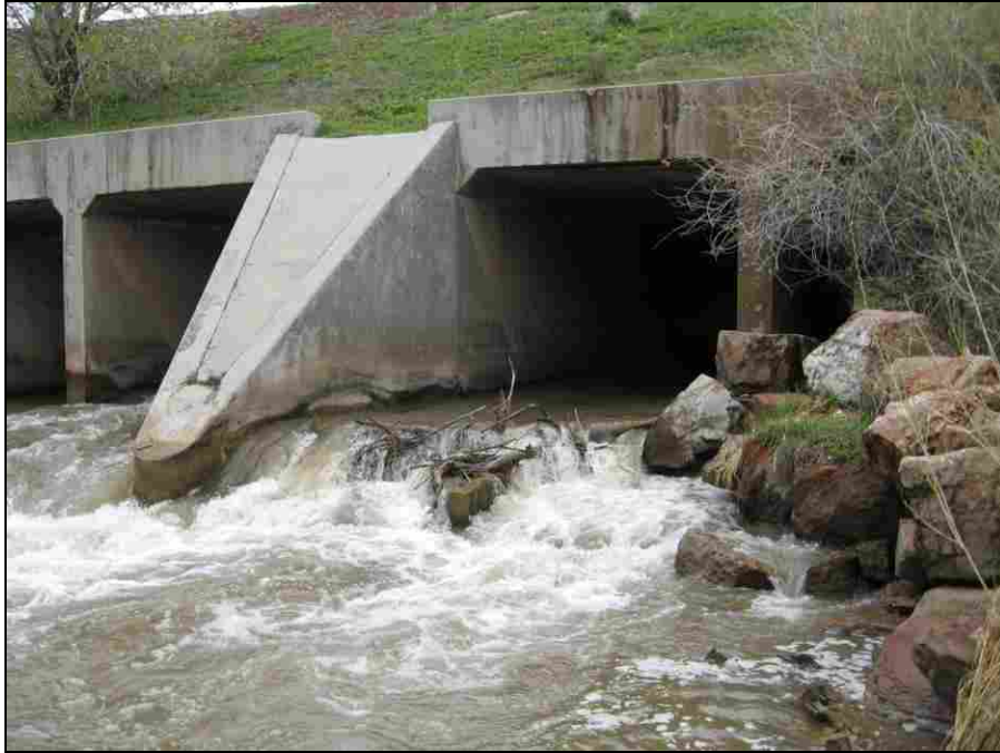
Figure 5-17: Debris Pile at Culvert Outlet
