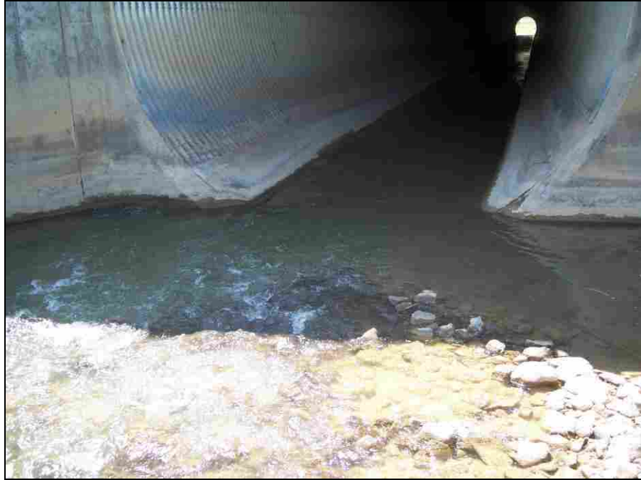
Figure 4-10: Inlet of Backwatered Culvert #2
