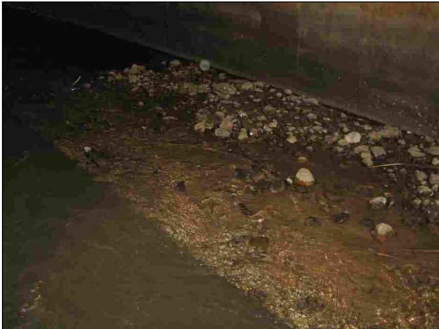
Figure 5-14: Fish Baffles Filled in With Sediment
