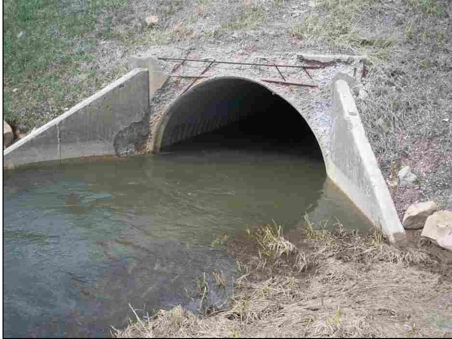
Figure 4-8: Inlet of Backwatered Culvert #1
