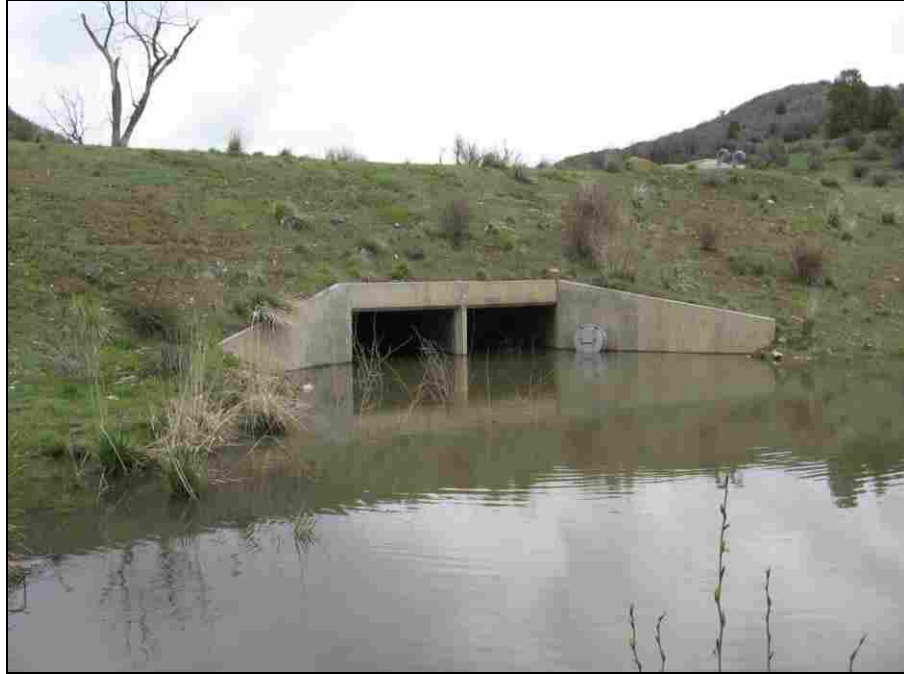
Figure 5-8: Backwater Conditions at Outlet Caused From Debris Dam
