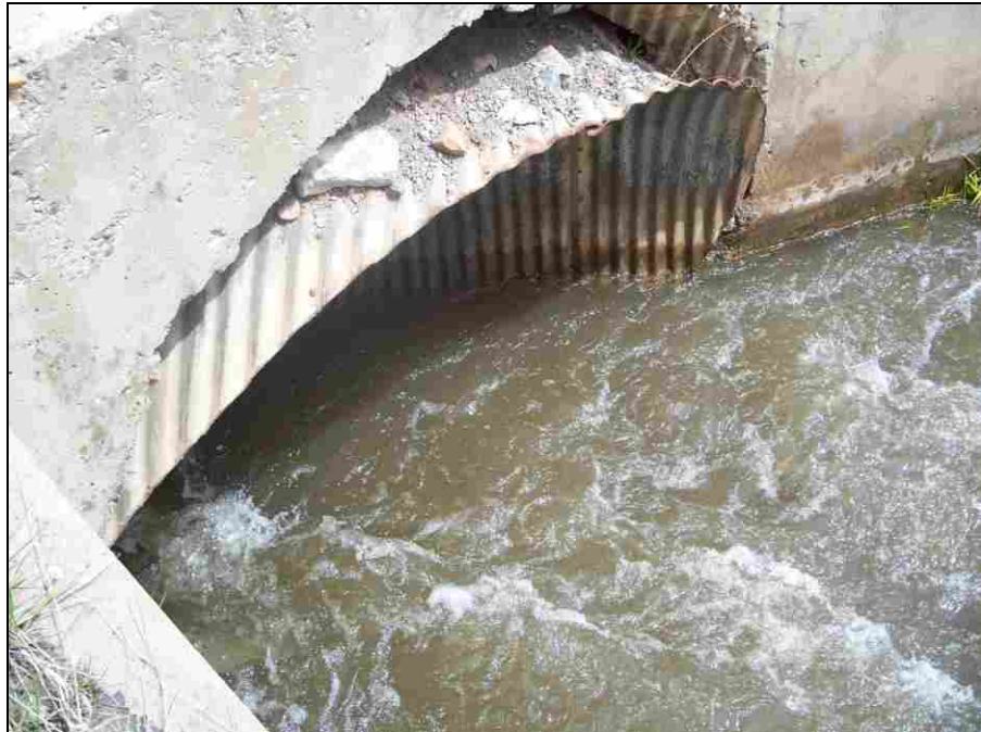
Figure 5-27: Culvert Separating from Headwall
