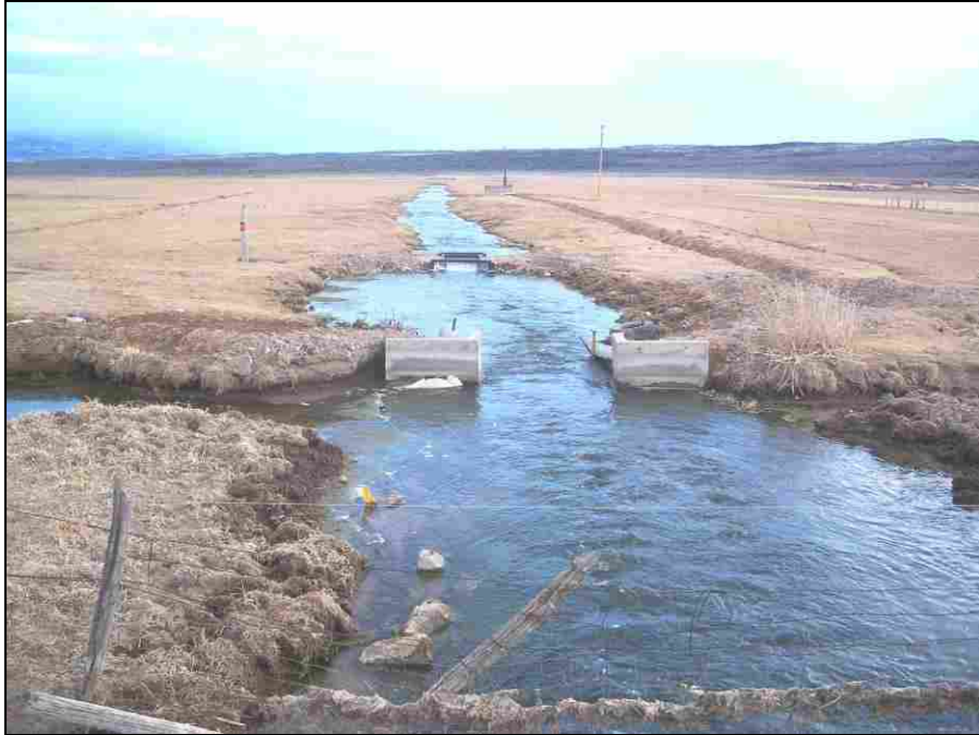
Figure 5-19: Two Small Diversions Within 100 ft. Downstream of a Culvert Outlet
