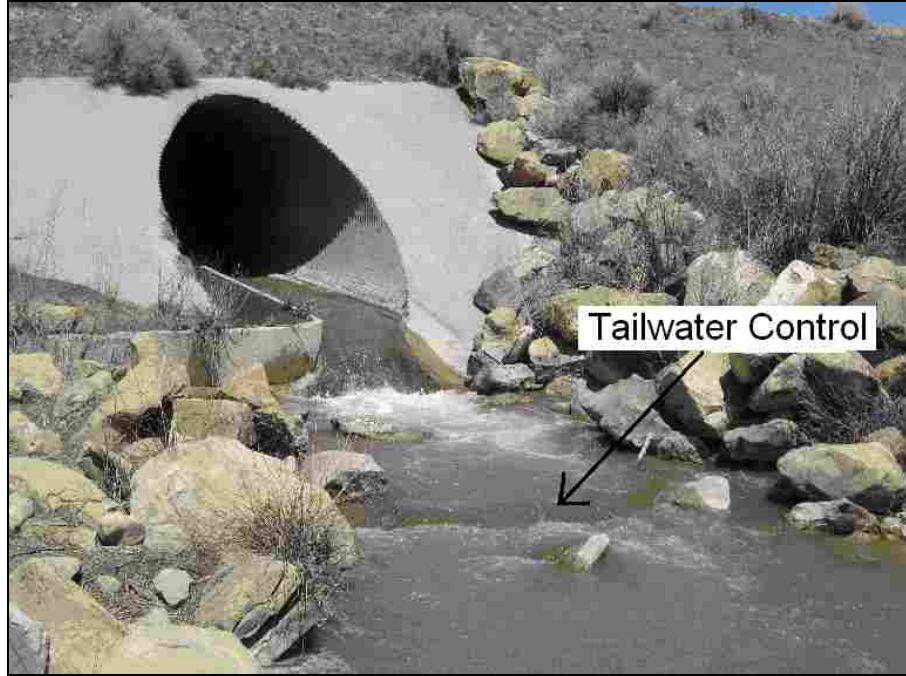
Figure 5-5: Outlet and Tailwater Control Photo
