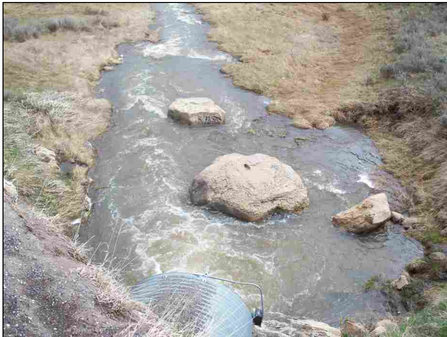
Figure 5-20: Large Boulders Downstream of a Culvert Outlet
