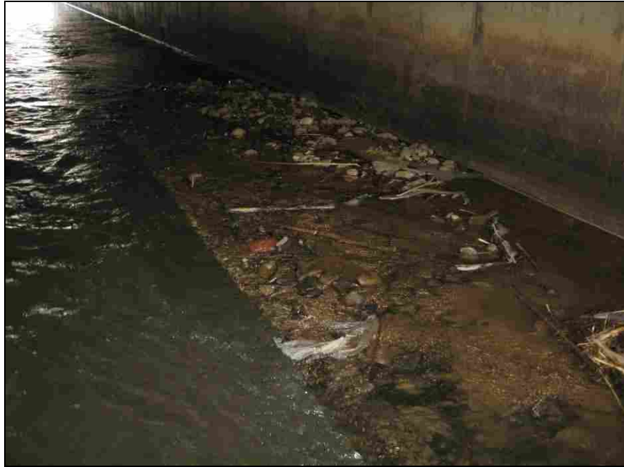
Figure 6-22: Close-up of Sediment Filled Section of Fish Baffles in Diamond Fork #2 Culvert
