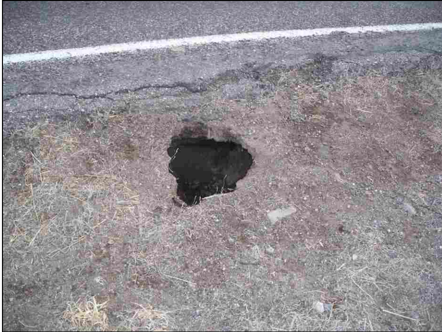
Figure 5-28: Possible Road-Side Erosion Associated with Figure 5-27
