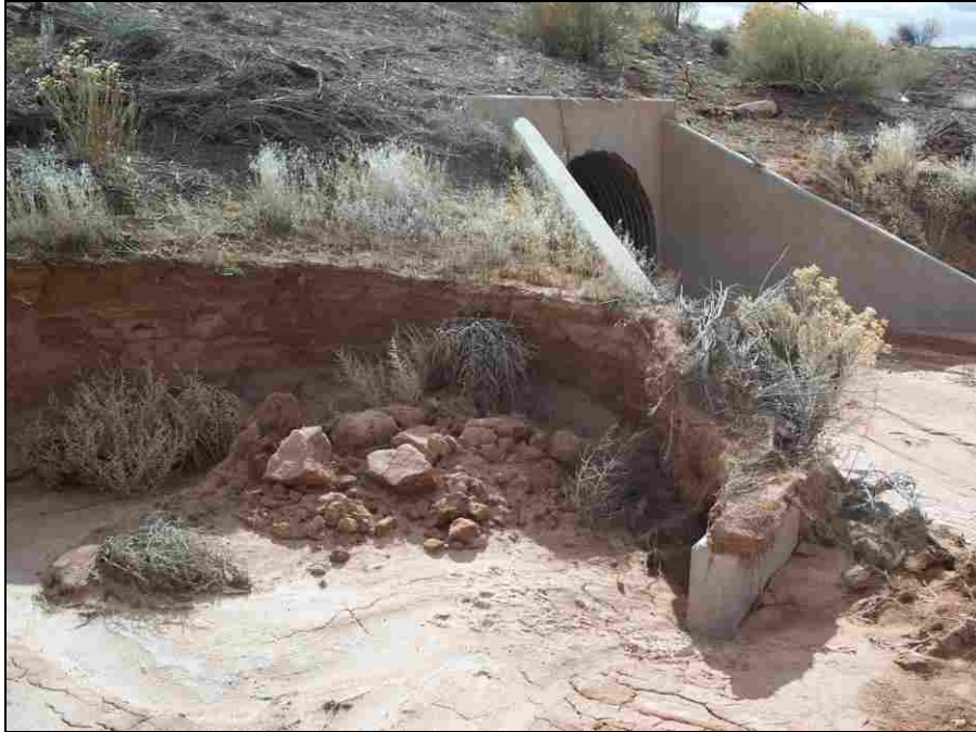
Figure 5-25: Erosion Behind Wingwall
