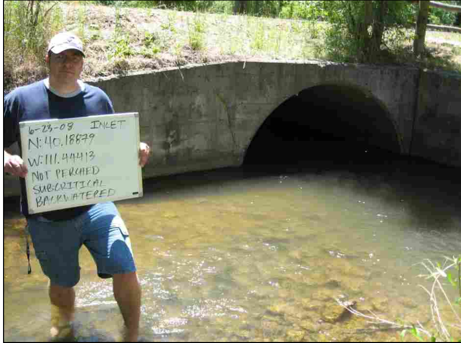
Figure 4-1: Hydraulic Evaluation Photo Taken at the Inlet
