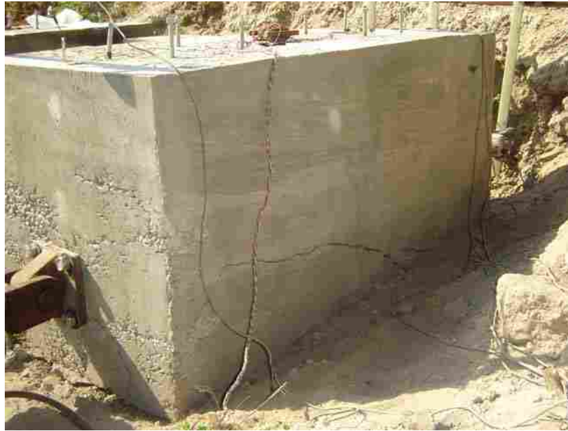
Figure 5-13 Cracking at a 90 kip load on the back and side of Test Cap 3.
