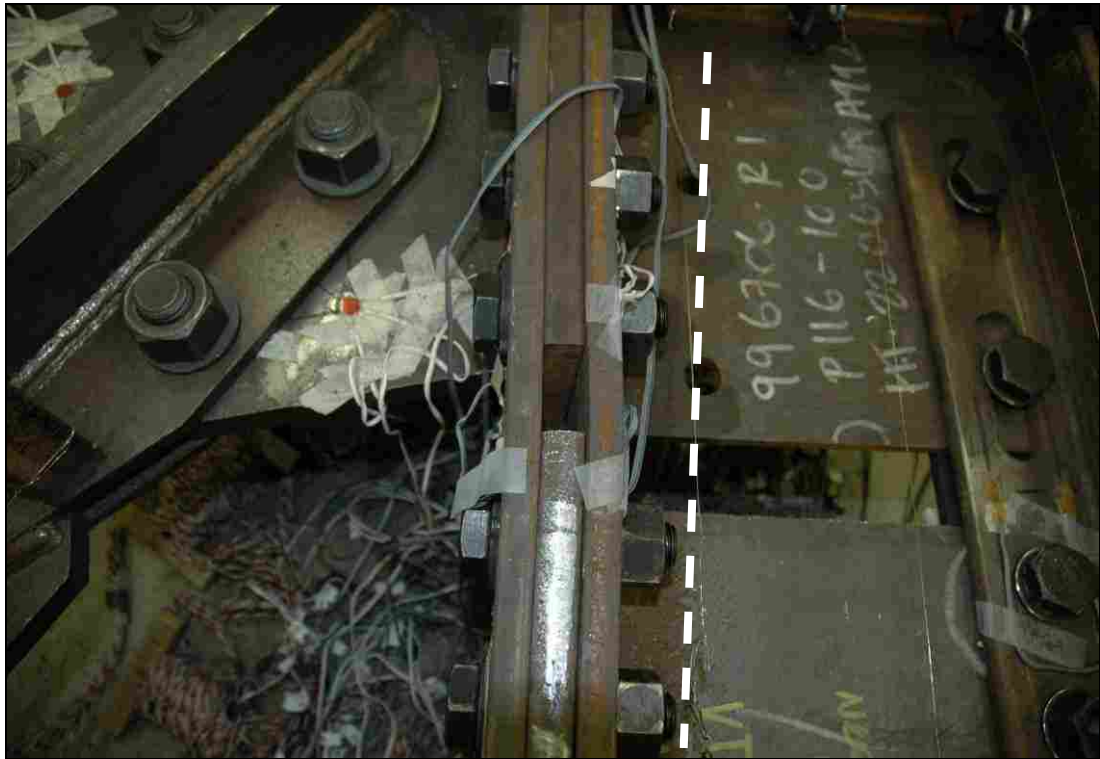
Figure 3-6 Specimen 1 – Splice Plate Deformation Following Boundary Failure
