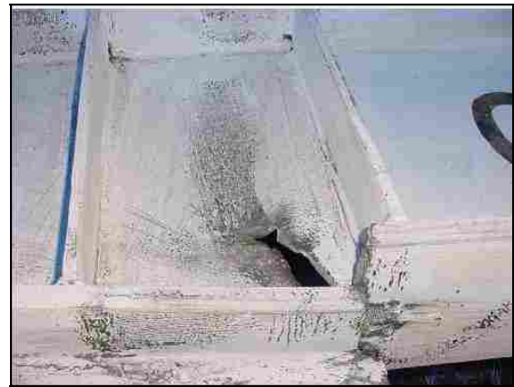
(b) Fracture of Beam Flange
