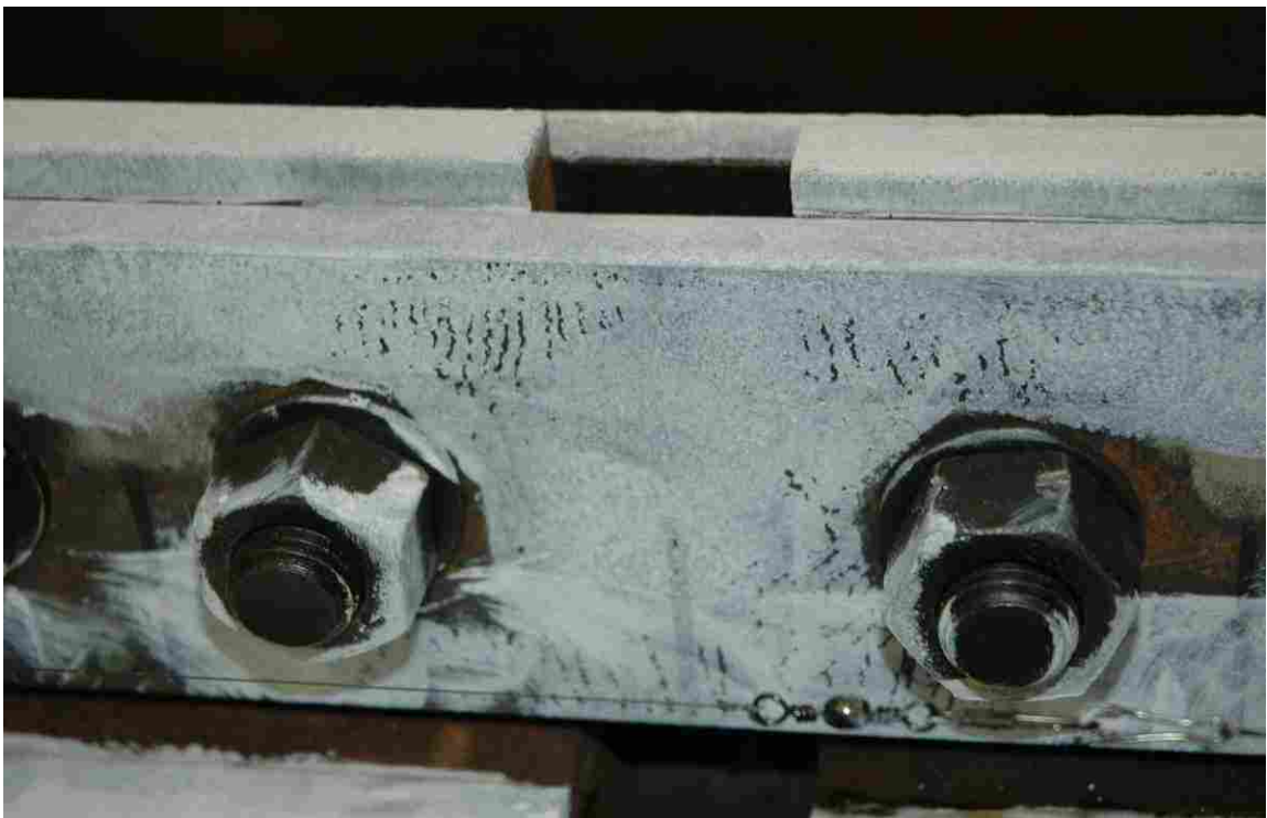
Figure 3-19 Specimen 2 – Initial Yielding of Splice Plate (2% Drift)
