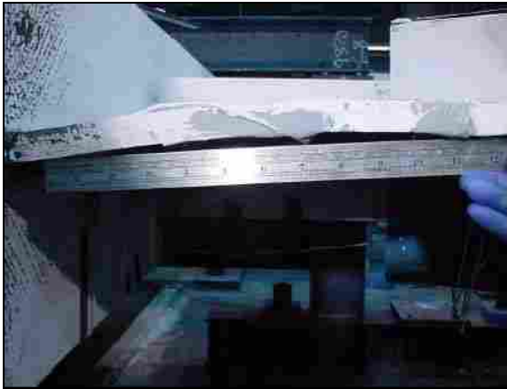
(a) Buckling of Gusset Plate
