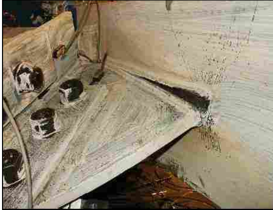
(a) Fracture of Gusset-to-Beam Weld
