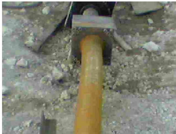
Figure 9-6 Picture of bent actuator extension.
