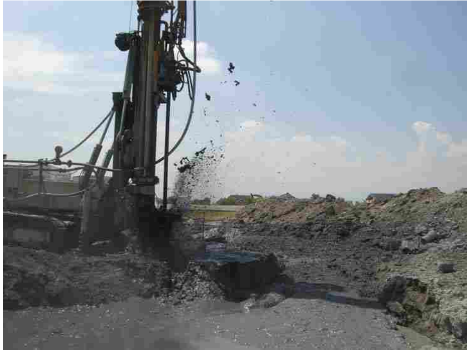
Figure 5-4 Photo of jet grout drill rig in position above buried foundation with spoil being ejected and washing down into the storage area.
