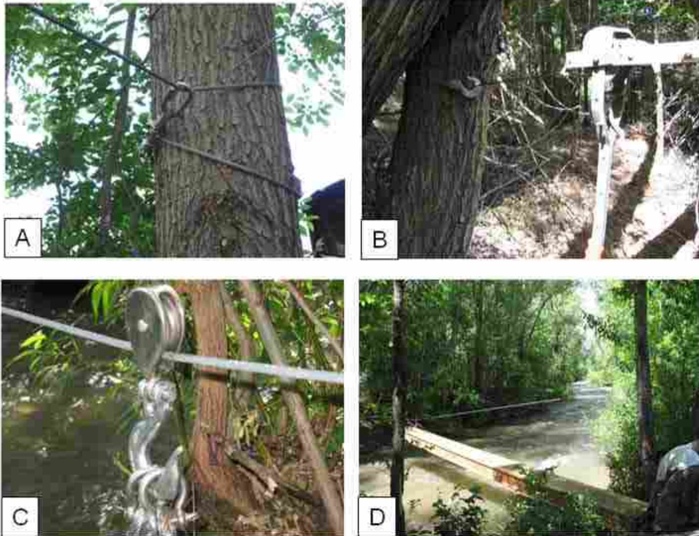
Figure A-14. A) Cable fastened around sturdy trees; B) hand winch used to tighten the cable; C) bridge is suspended by pulley, D) and pushed across the stream.
