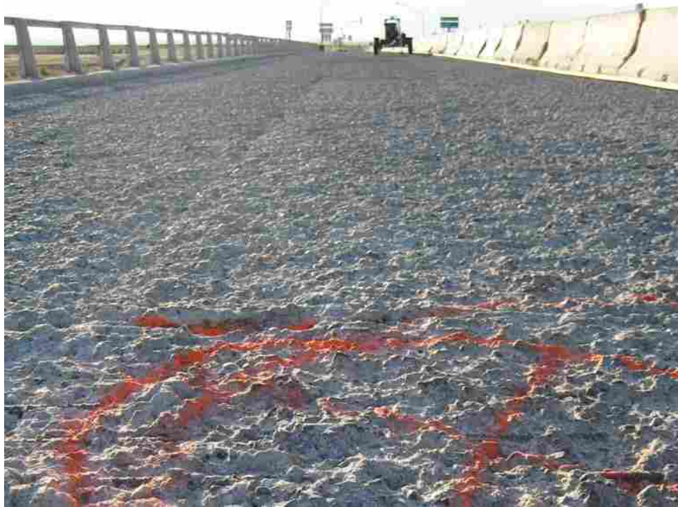
FIGURE 2.5 Rough surface for bonding of new overlay.
