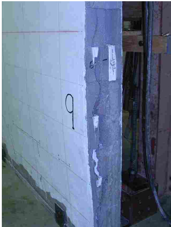
Figure 6.6 Cracks Separating Grouted and UngROUTED Faces of the Blocks
