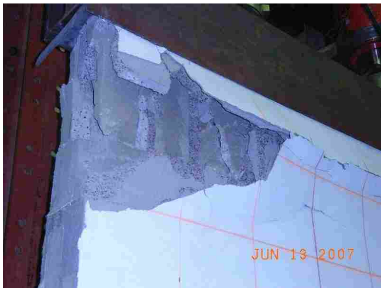
Close-up of Failed Section (wall #1)
