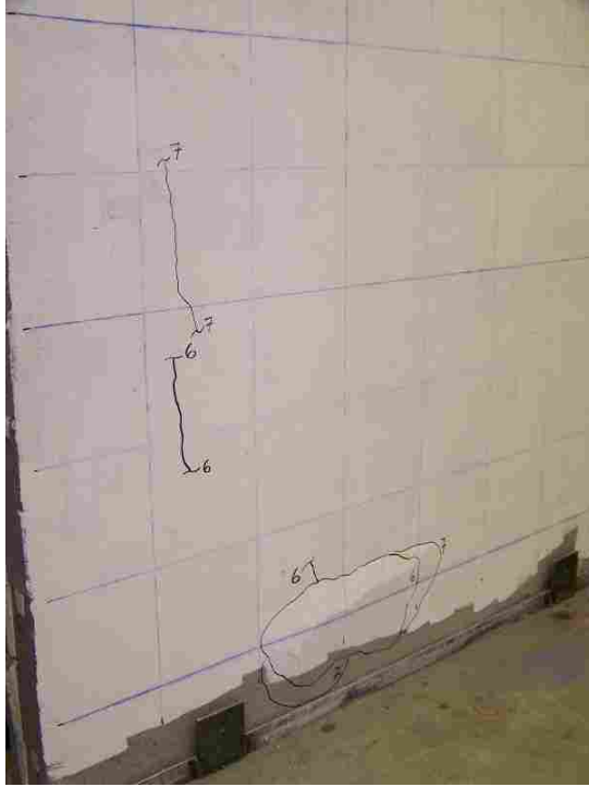
Buckling of Structure Coat at Bottom of Wall (wall #3)
