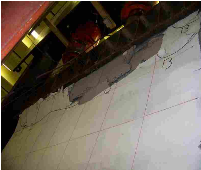
Failure at Top Course of Wall (wall #5)
