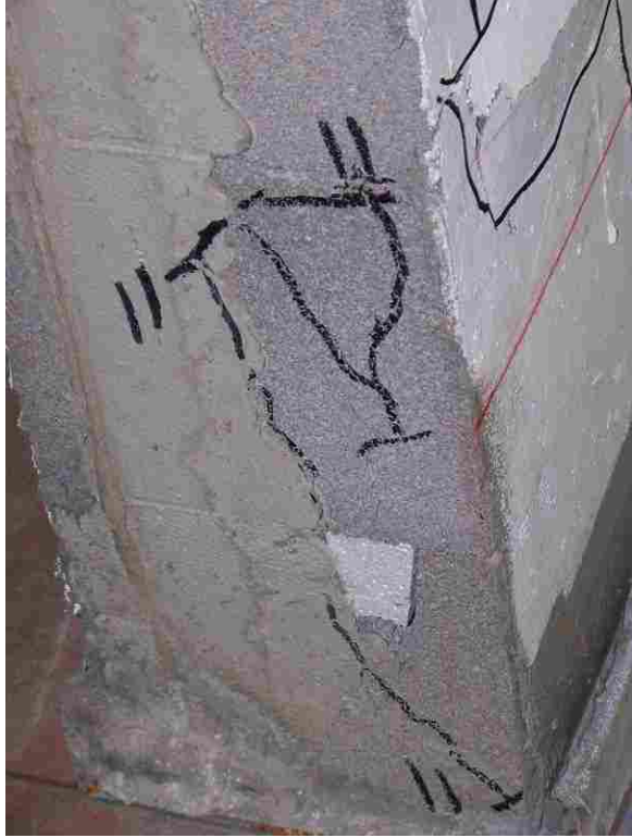
Cracking at Side of Wall (wall #5)
