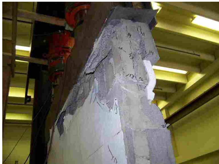
Close-up View of Failed Section (wall #2)
