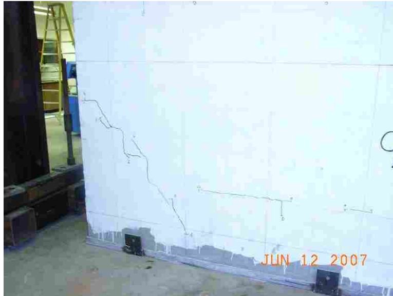
Diagonal Cracking at East Side of Wall (wall #9)
