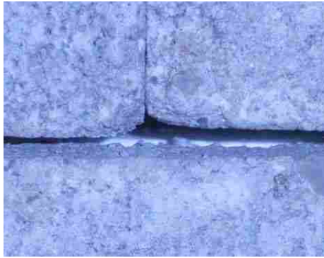
Figure 4.2 Gap in Wall Created by Non-Uniform Block Heights
