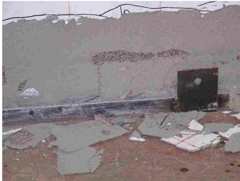
Separation of Structure Coat at Failure (wall #2)
