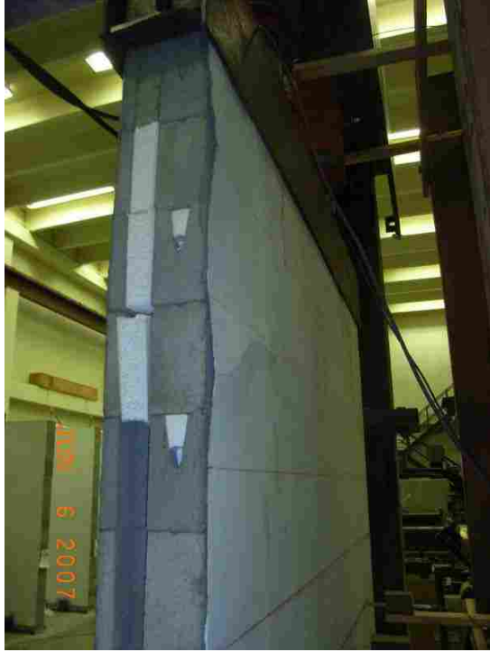
Bubbling of Structure Coat (wall #10)
