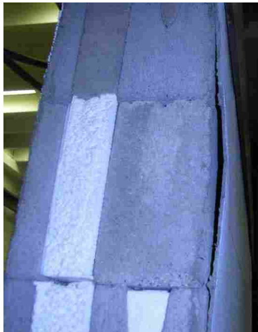
Figure 6.2 Bubbling of Structural Coating
