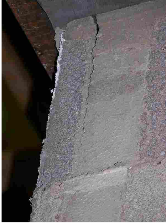
Cracking at Side of Wall (wall #5)
