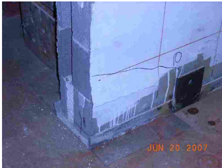
Damage at East Corner Possibly Due to Low Spot in Floor (wall #7)
