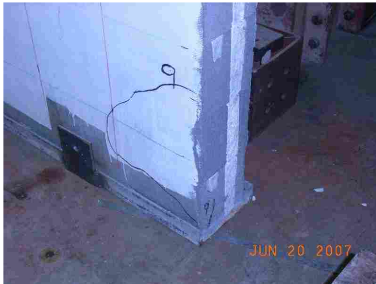
Damage at Lower West Corner (wall #6)
