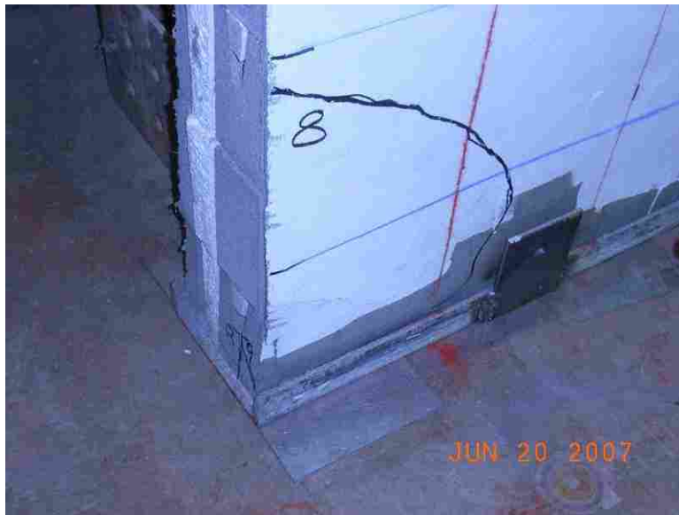
Damage at Lower East Corner (wall #6)
