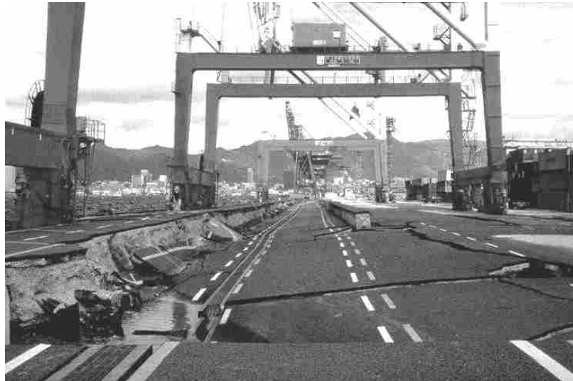
Figure 1-2: Lateral spreading on Port Island, Japan, 1995 (U of W, 2000)
