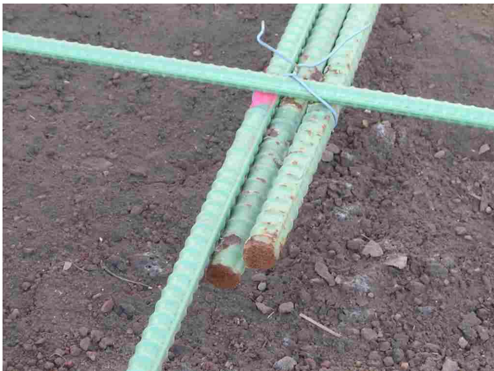
FIGURE 2.1 End cut damage in the field.
