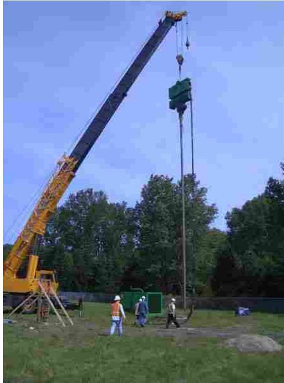
Figure 4.2 Drain installation was accomplished with the use of a 70 ton crane and a vibratory hammer and mandrel.
