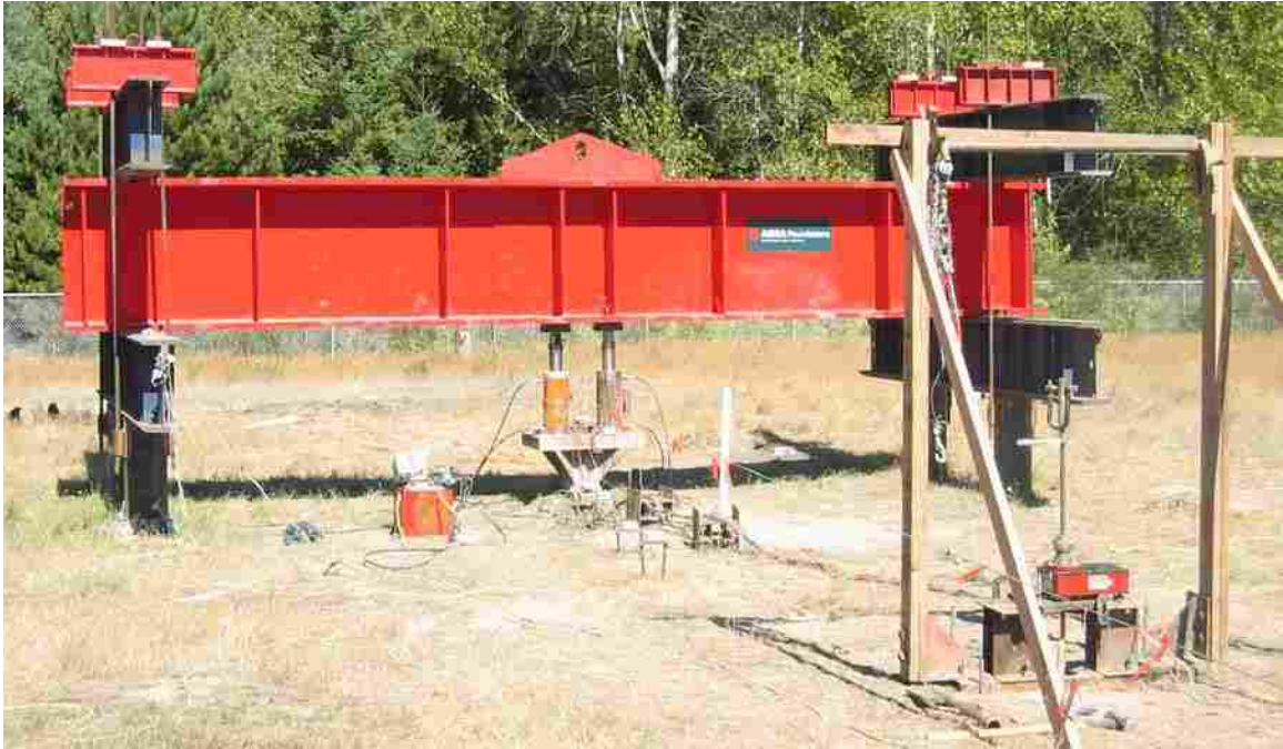
Figure 5.10 Photograph of the completed test frame. The wooden frame in the foreground was part of the test apparatus involved with the vane shear test.
