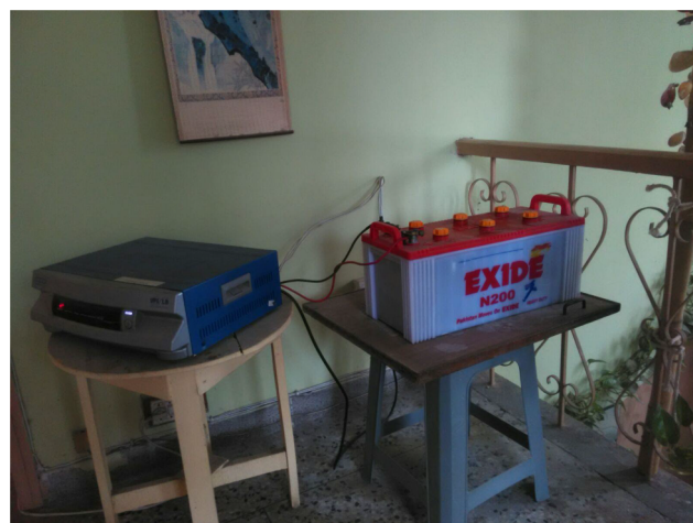
Fig. 2. UPS and battery – photograph by Ayah.
