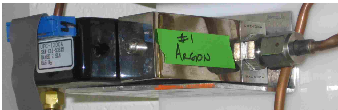
Figure 2.6 Mass Flow Controller used to control the argon flow.
