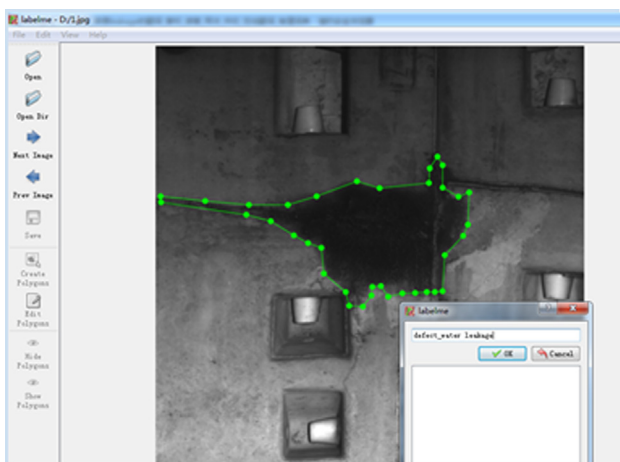
Fig. 3. Moisture marks annotated by LabelMe.
